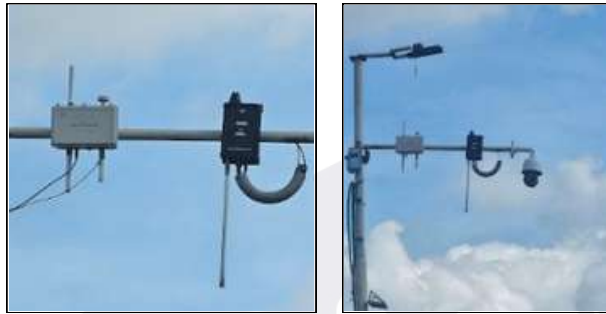
Figure 5. OBU, RSU pole deployment
