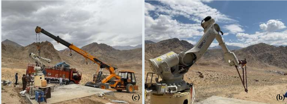
Fig 3: (a) Schematic of the robotic arm printing system; (b) The robotic-arm printing system being off-loaded on site; (c) Installation and operation of the robotic arm system in Leh.
