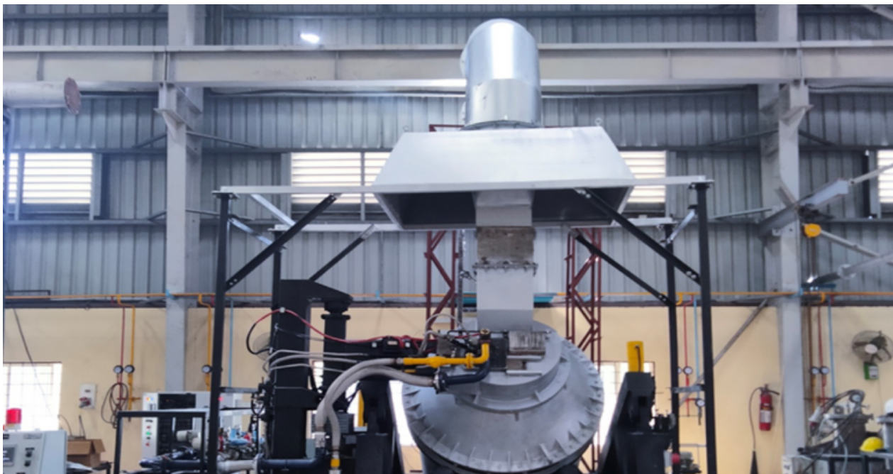
Fig. 2a): Rotary tilting furnace for PCB recycling
